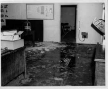
05.Warehouse after rain
